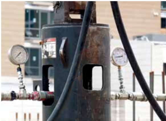
Figure 2.12.2.3.a1 Dual pressure gauges
