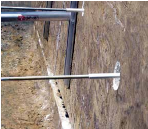
Figure 4.2.5.1.b1 Before: Shear movement of a block wall evident from exterior
