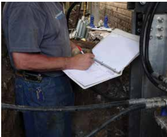
Figure 3.10.m Pressure readings are recorded for each pier tube
