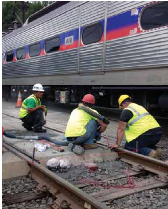
Figure 5.3.a1 Commuter train track settled up to 2 inches at intersection
