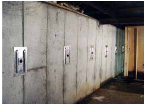
Figure 4.2.5.1.a2 After: Wall is immediately returned to original straight position after backfill soil is removed and Geo-Lock anchors installed
