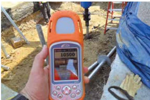
Figure 2.12.2.3.e2 Torque transducer providing direct reading of torque for helical pile project at Reagan National Airport
