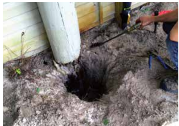
Figure 5.2.f PolyLEVEL resin stabilizes loose sand to prevent undermining of slab during column repair
