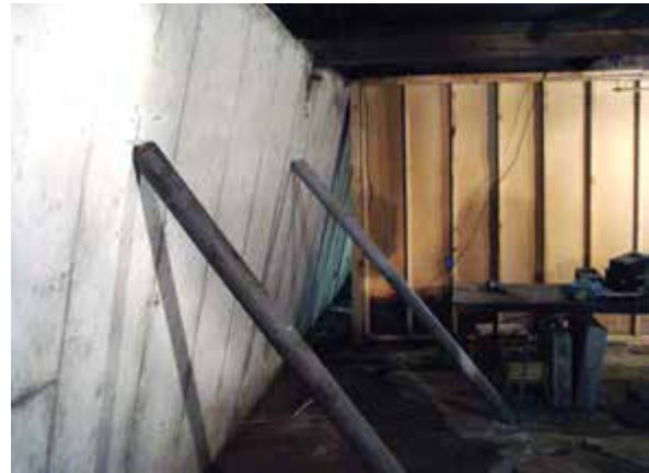
Figure 4.2.5.1.a1 Before: Poured concrete basement wall severely leaning in at the top
