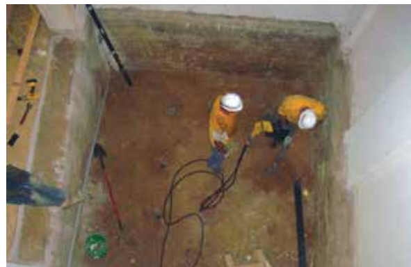
Figure 2.4.a3 Helical piles installed with hand-held equipment to support new elevator within existing school
