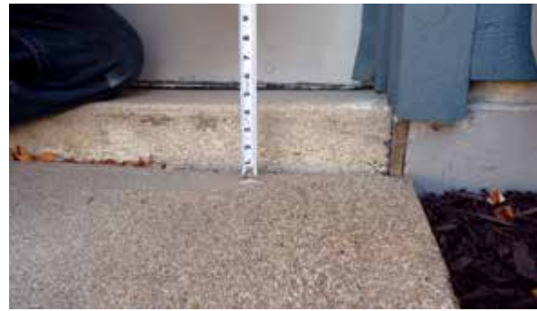
Figure 5.2.b1 Before: Driveway settled up to 4 inches relative to garage slab
