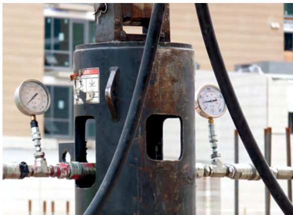
Figure 2.12.2.3.a1 Dual pressure gauges
